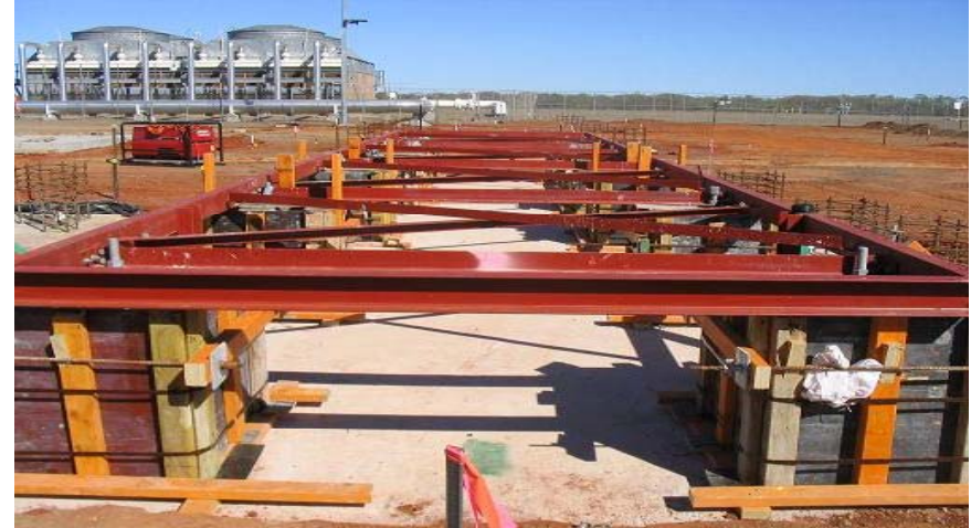
CS3 Compressor/Turbine Base and Pedestals
